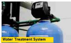
Water Treatment System
